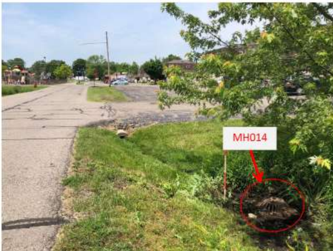
Google street view image taken in August 2018 of Schroeder Blvd., facing west and showing the location of the manhole recommended to repair.
