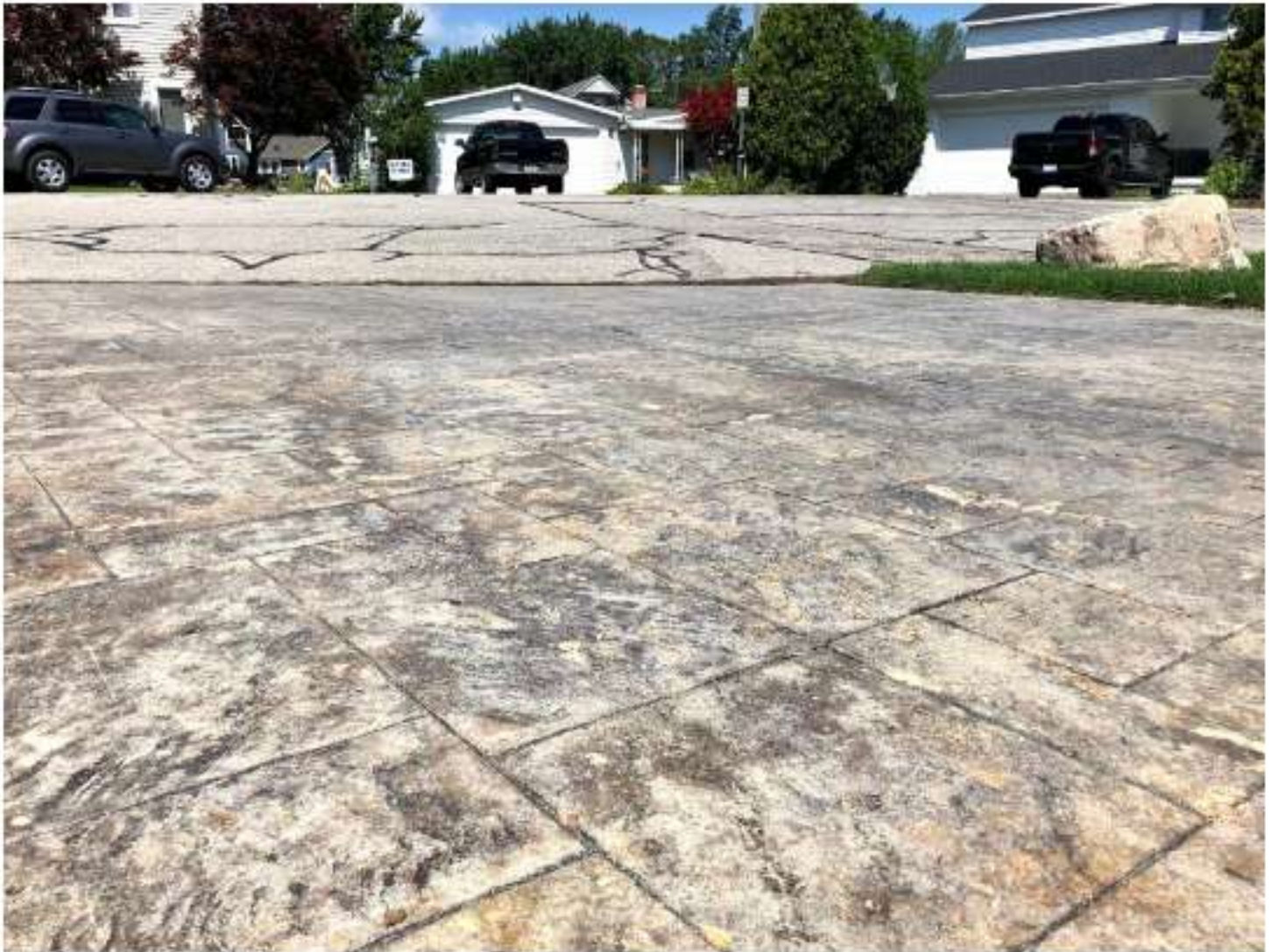
Elevation comparison of driveway compared to the road from July 30, 2019, taken by HRC staff.
