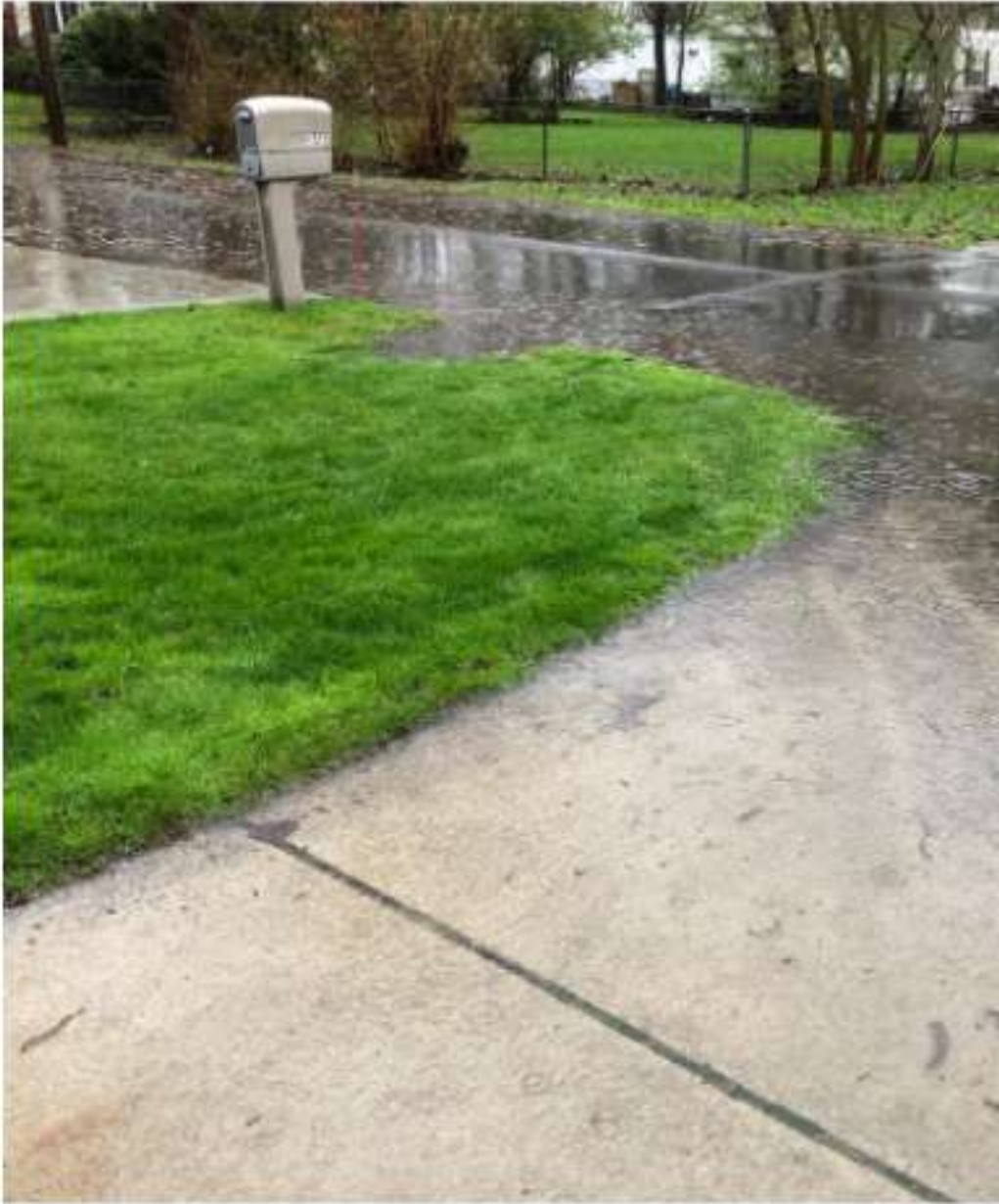
Photo from homeowner at 2229 Willow Beach St from May, 2019 of the flooded driveway and street.
