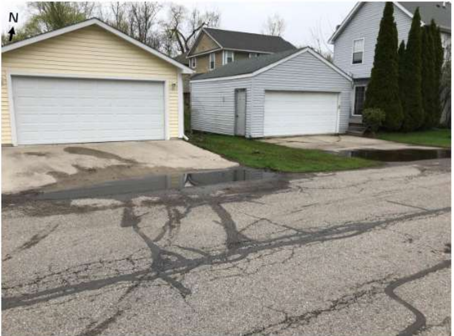
Image taken by HRC staff on May 3, 2019 of standing water at driveways of 2141 Willow Beach Street and 2140 Brock Street.
