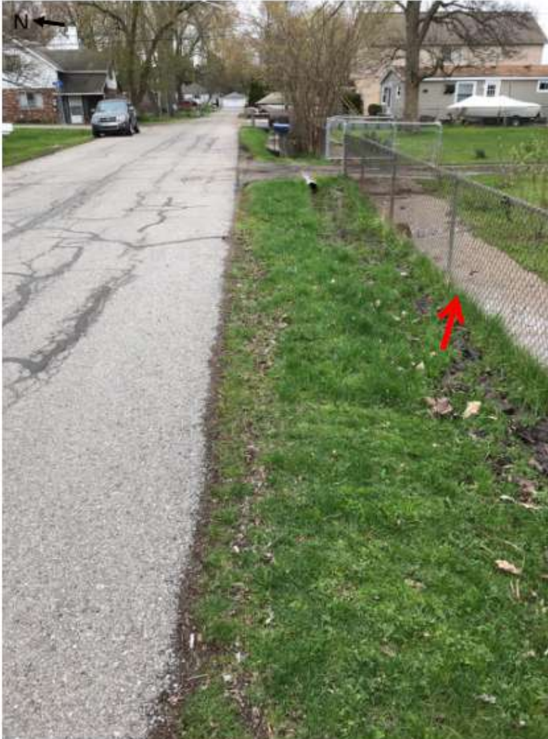
Image taken by HRC staff on May 3, 2019 of the heaved culvert at 3201 Kenrick and the location where the homeowner of 3201 Kenrick placed a sand berm to prevent roadway runoff from draining to their property.
