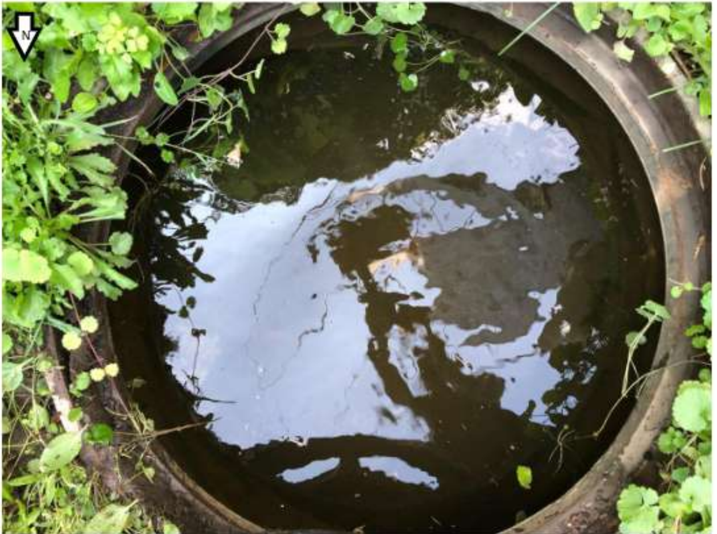
Inside image of the manhole at the end of Maddy Ln that is regularly filled with water as the outgoing pipe is below the water level in the stream.
