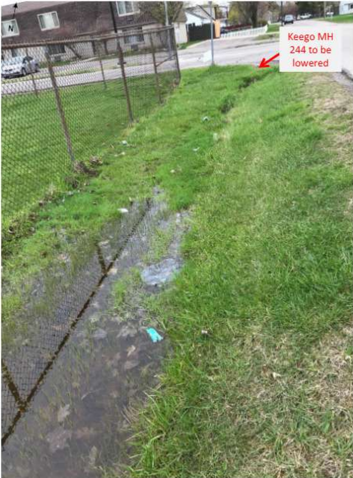
Photo taken by HRC staff on May 3, 2019 of stagnant water in the ditch along Beechmont, south of Schroeder, that's prevent flow from entering the manhole.
