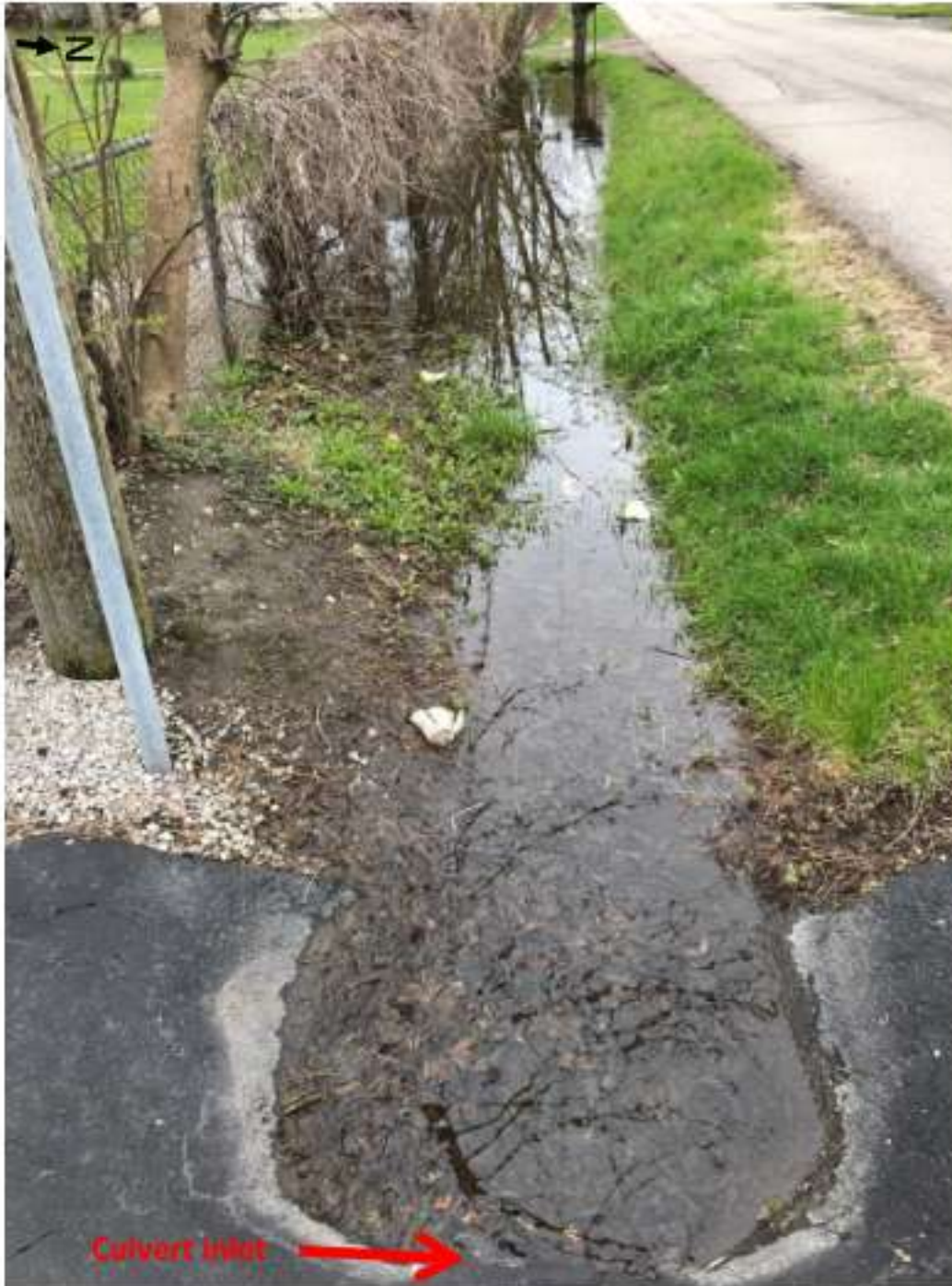
Photo taken by HRC staff on May 3, 2019 of clogged culvert inlet and stagnate water at 3185 Kenrick Street.
