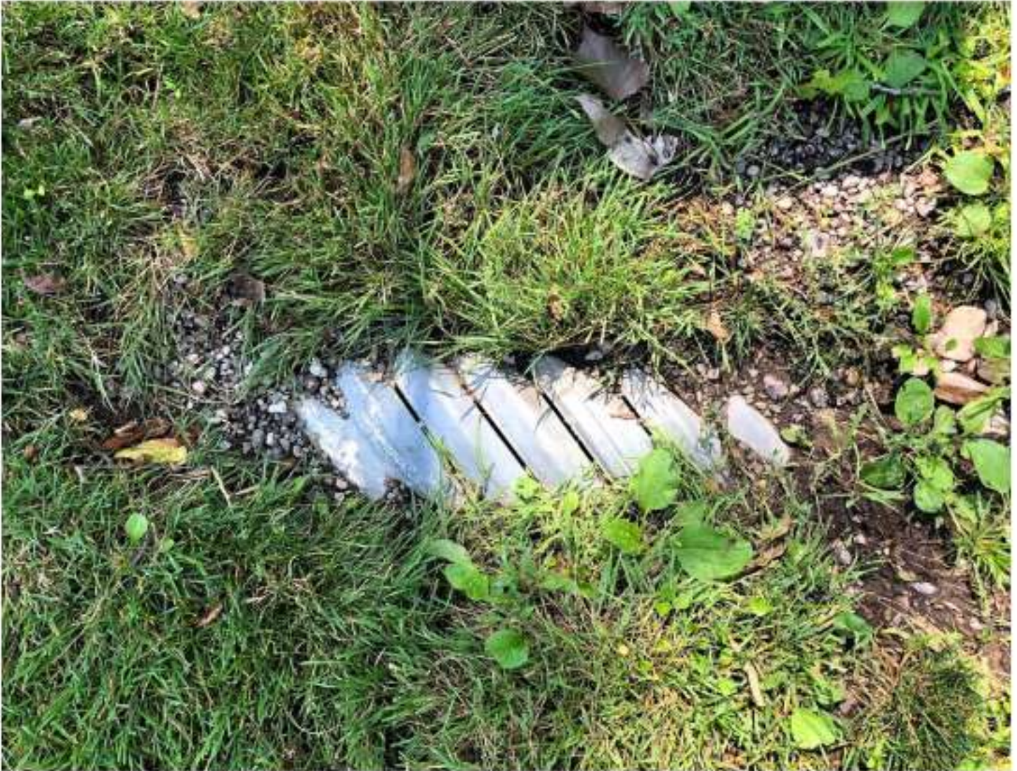
Photo taken by HRC staff the exposed drain and slit created to allow flow into the pipe from July 30, 2019. Location where field catch basin is recommended to be installed.
