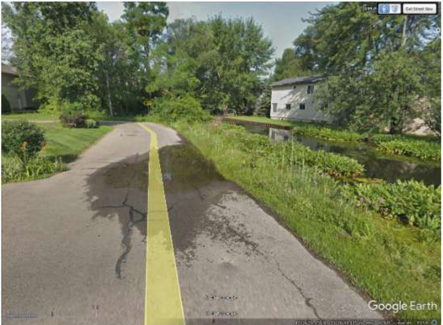
August 2018 Google street view image of low-lying area in front of 3119 Brock Street that experiences frequent water ponding.
